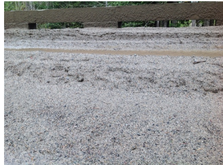
sediment on deck
